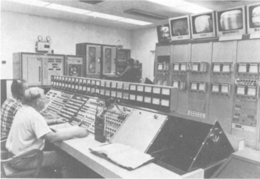
FIGURE 20-3. Control room (inside a reinforced concrete blockhouse) for test operators, instrument recorders, and controls. Note the control console, closed-circuit television, radio and telephone, direct read-out meters, strip charts, high-speed tape recorders, oscilloscope, air-quality alarm, and emergency lights. (Courtesy of U.S. Air Force Phillips Laboratory.)
